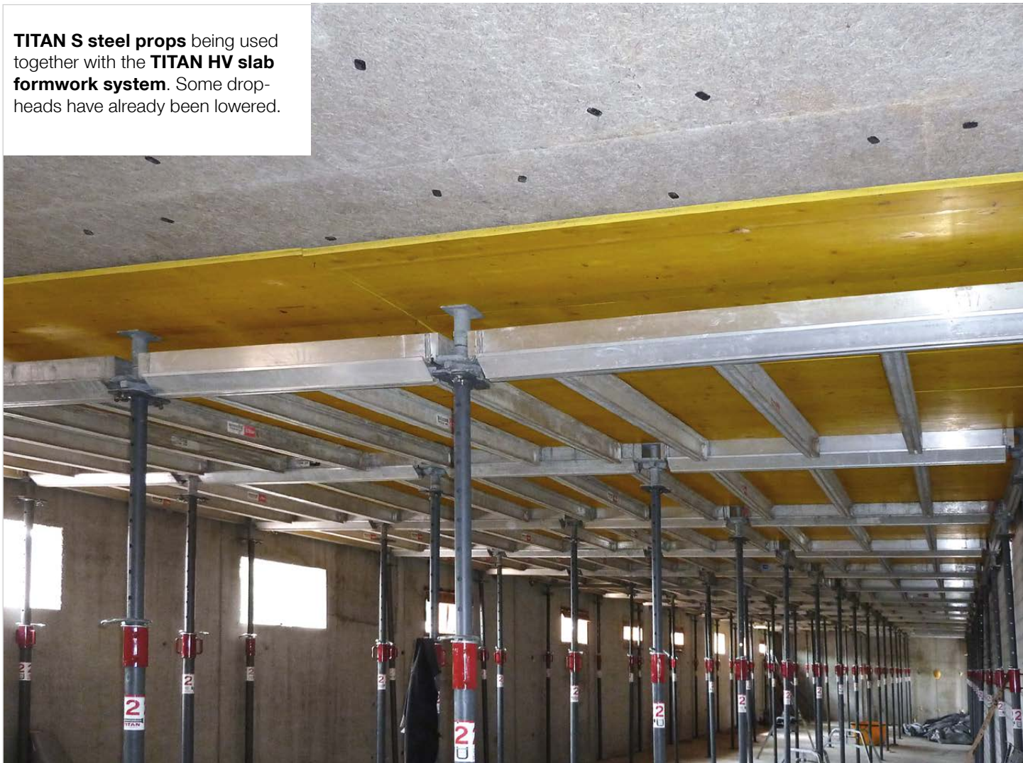
TITAN S steel props being used together with TITAN 120 aluminium formwork beams to support a floor of precast elements + in situ topping over a basement.
